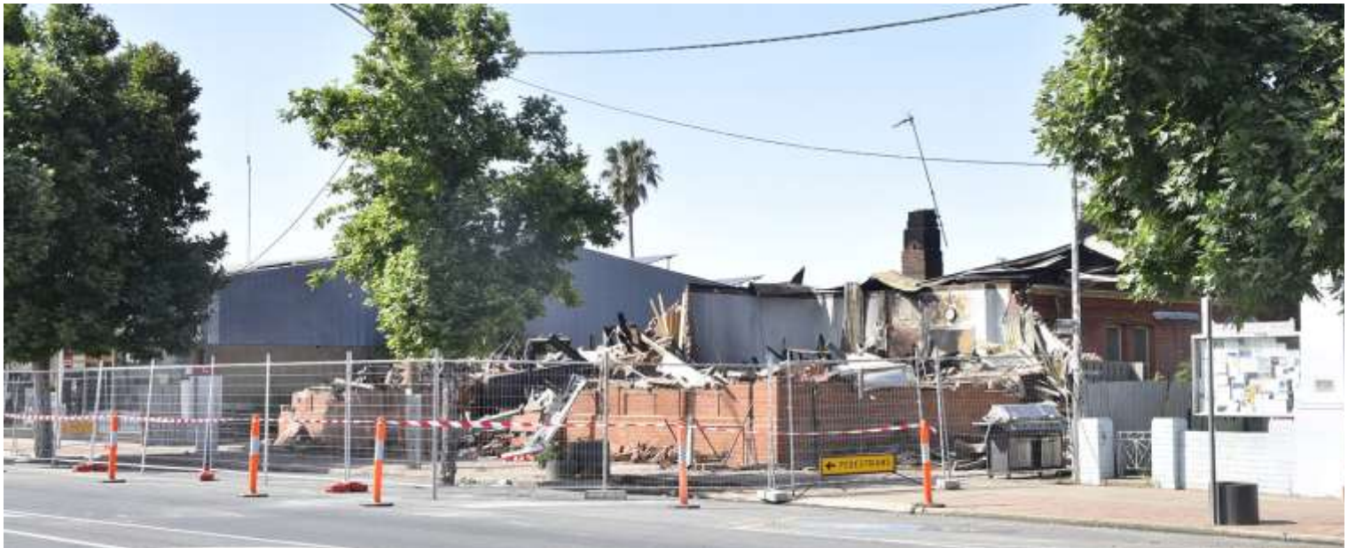
A sad sight in the main street – the aftermath of the fire.
