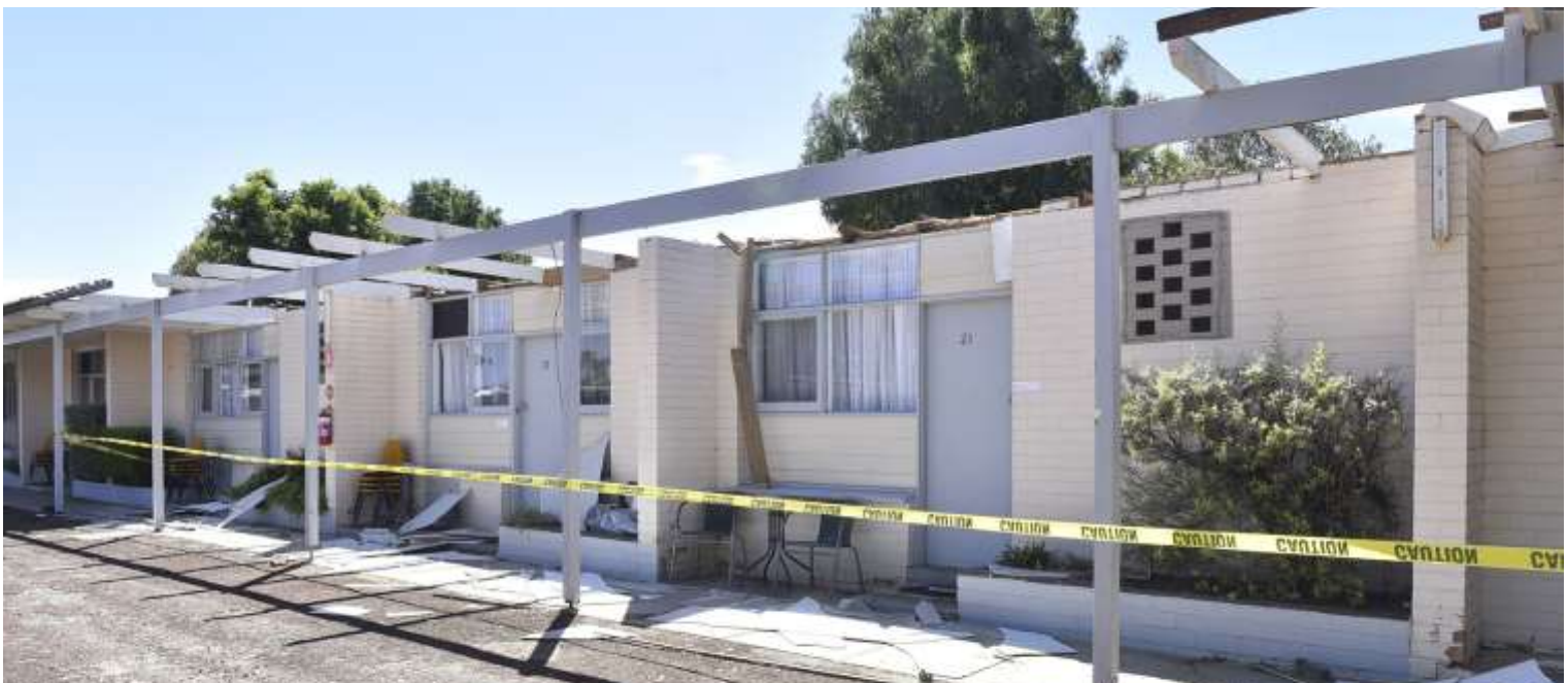
The Charlton Motel sustained damage to five units during the storm.
